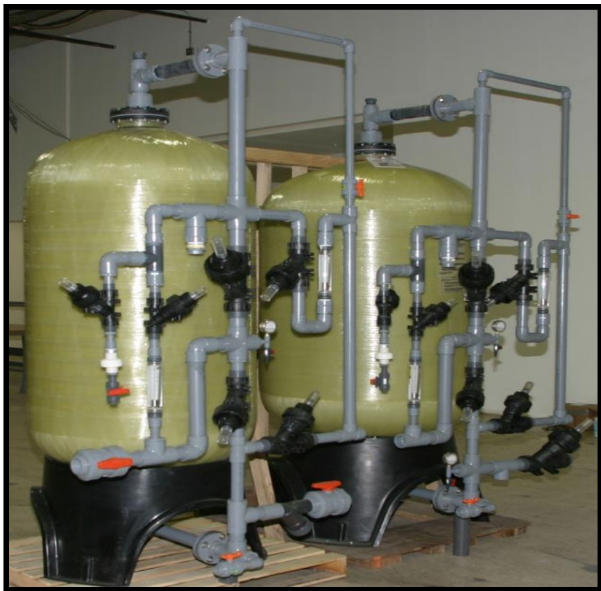
DEIONIZED WATER PLANT
